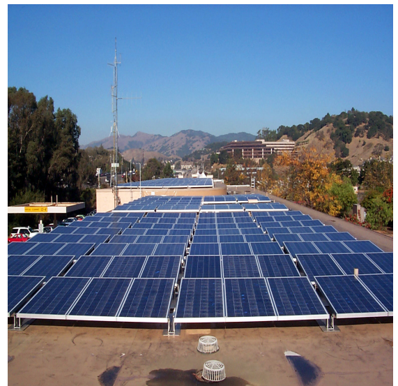
89 kilowatt solar rooftop installation at the General Services Building in Marin County.
