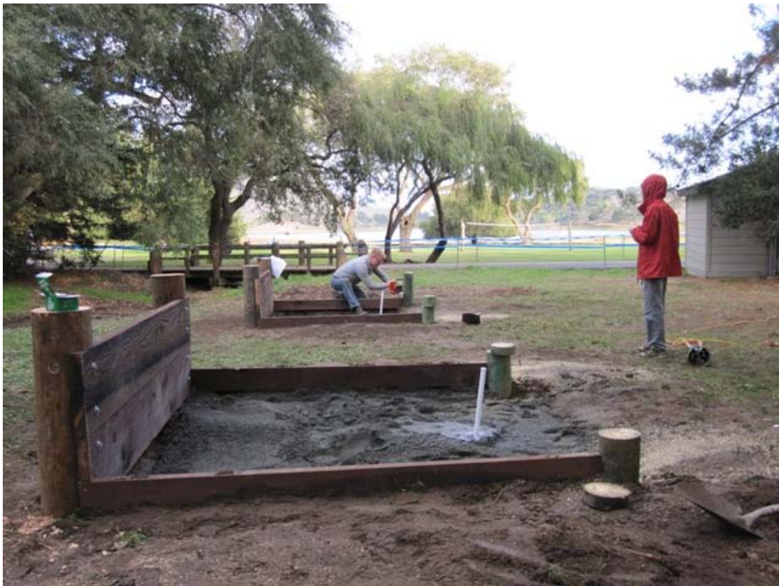
Scoutmaster and General Contractor 'Eric' helped lead a troop of boy scouts in re-constructing the Area 1 horseshoe pits at Stafford Lake Park on November 6 th , 2011.
